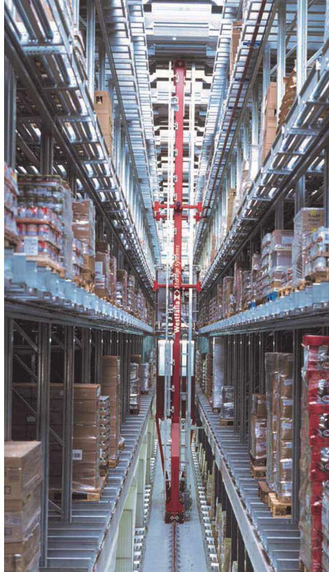
High Cube Warehouses utilize automated storage and retrieval systems (ASRS) to move and retrieve goods. Photo Courtesy of Westphalia Technologies, INC.
